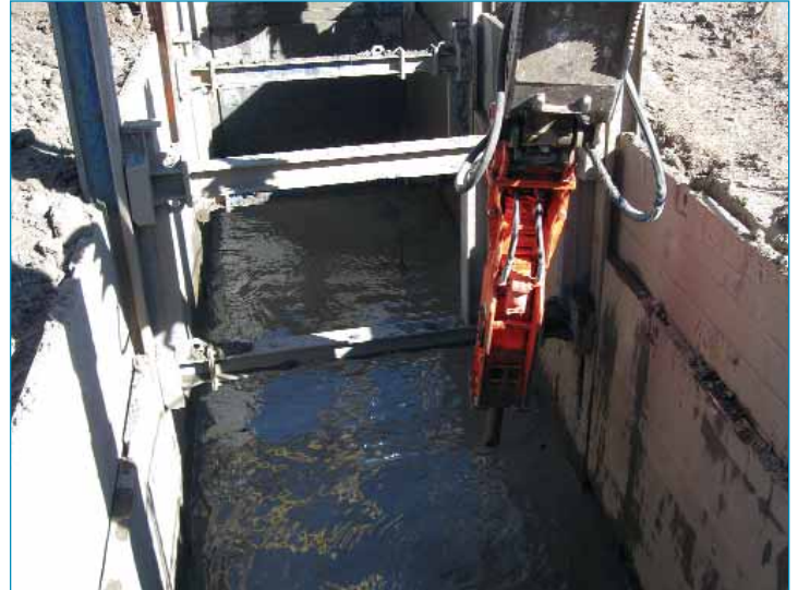
IWS encounters shallow groundwater in shoring structure. Jack hammer is breaking up bedrock.
