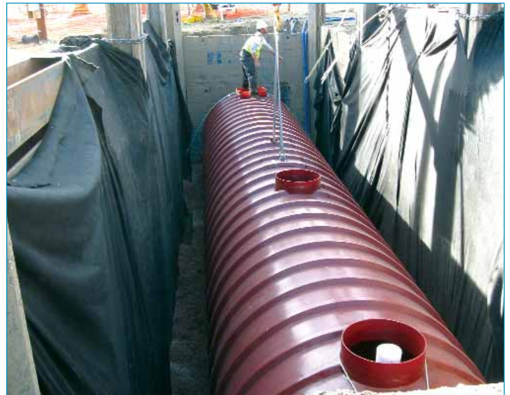
IWS setting tank in shored structure
