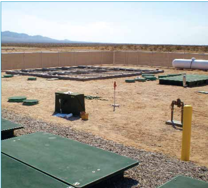
Advantex in foreground and Upflow Filter in corner
