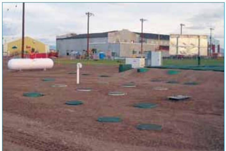
View of the completed treatment system
