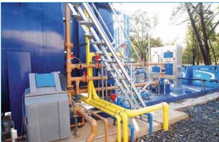
Chemical feed and associated piping for MBR
