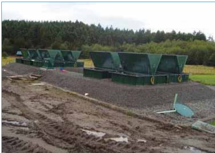
Advantex pods installed on top of existing sand filter
