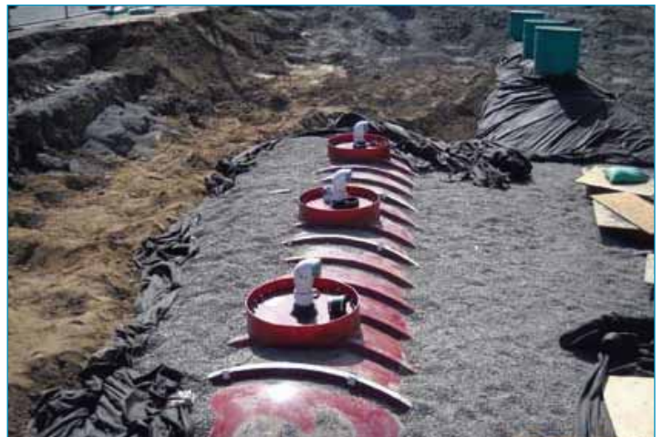
IWS Upflow Filter installed in tank below grade
