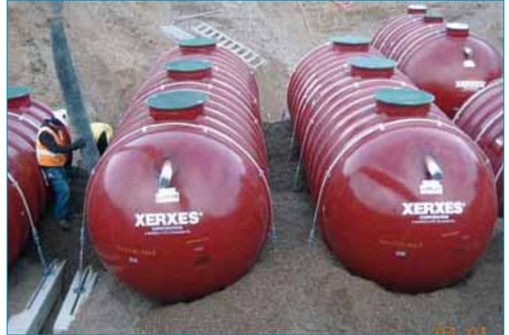
The two center tanks are the IWS Upflow Filters
