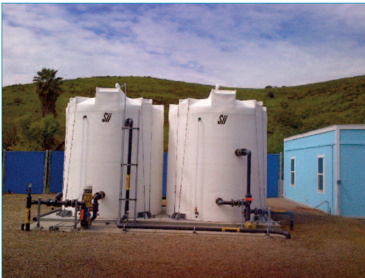
Pre-Chlorine Contact Tank and RO Product Tank
