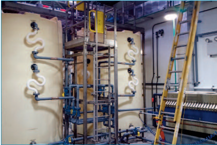
Waste Activated Sludge (WAS) Tanks
