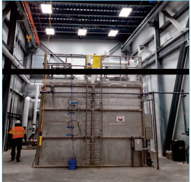
Membrane Bio Reactor (MBR) Unit
