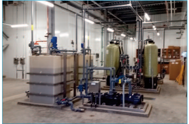
Ion Exchange Treatment
