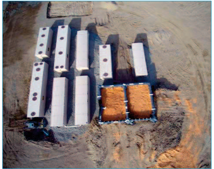
Arial View of Wastewater Treatment
