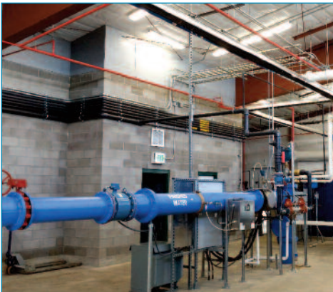
Finished Water Service with UV System and Blowers in background
