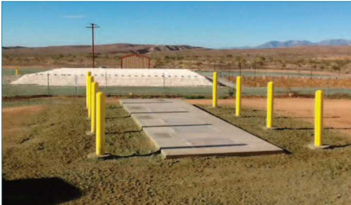
Completed Treatment System – Primary Tank, Anoxic Wetland, and Drain Field
