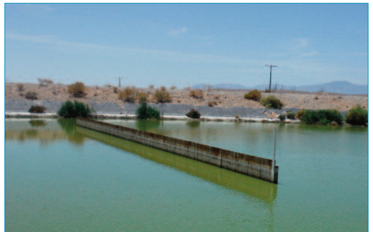
Evaporative Pond with a foot of sludge at the bottom that needed to be dewatered and disposed of
