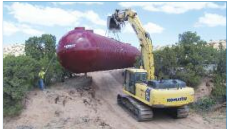
Walking one of the Xerxes treatment tanks
