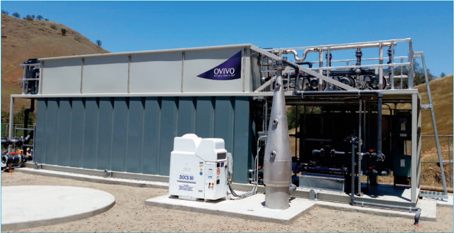
microBLOX unit installed
