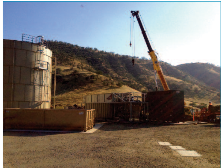
Water Tank, microBlox, and Generator
