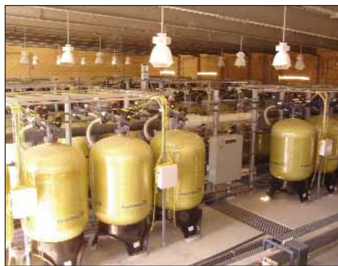
Completed Ion Exchange Treatment Trains
