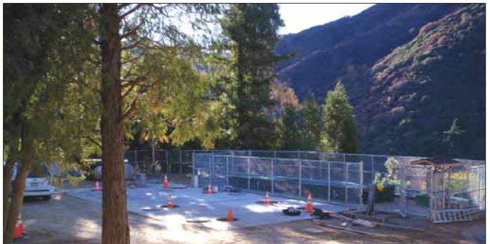
The new wastewater system included primary and secondary treatment
