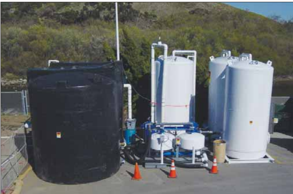
Pure Effect Dewatering Treatment Train
