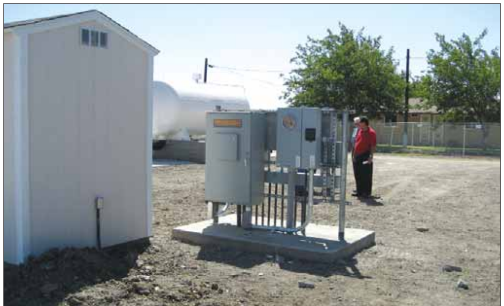
Reconfigured electrical and programmable control system
