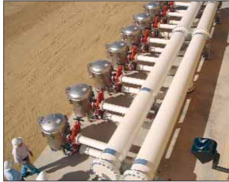
Pre-filters and Influent Manifold Assemblies
