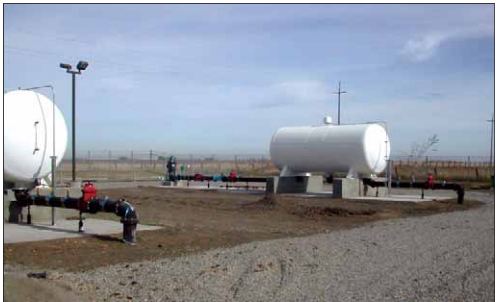
5,000 gallon hydronematic water storage and distribution tanks
