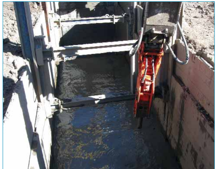
IWS encounters shallow groundwater in shoring structure. Jack hammer is breaking up bedrock.
