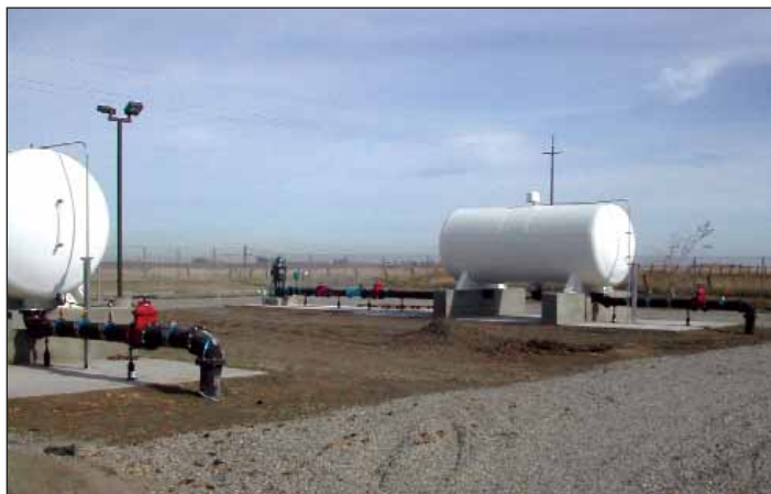
5,000 gallon hydropneumatic water storage and distribution tanks
