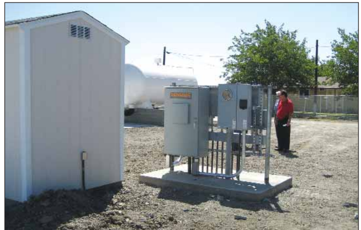
Reconfigured electrical and programmable control system
