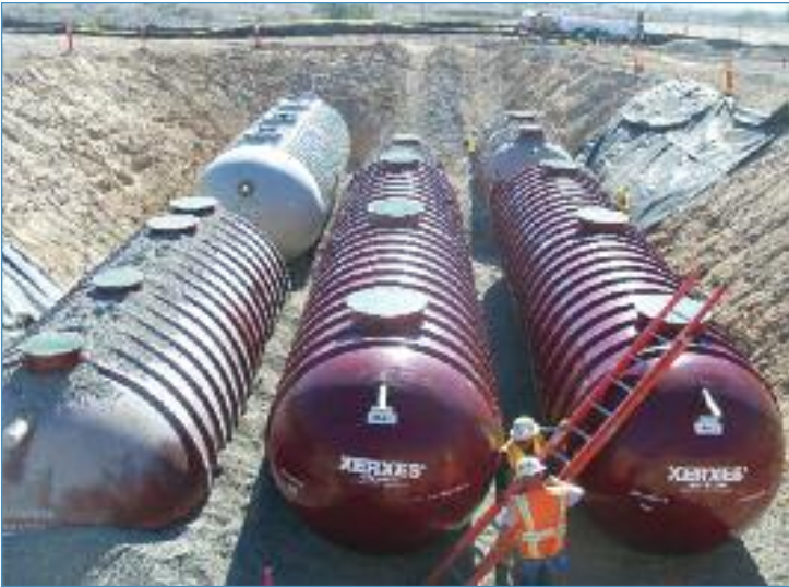
The two ENR Denite units are set in the foreground in the Xerxes tanks
