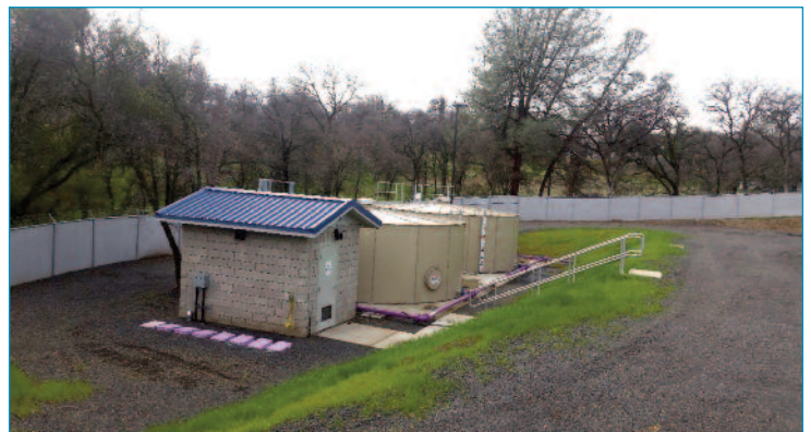
Storage Tanks and Pump House
