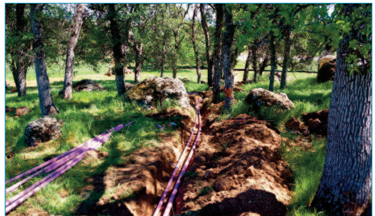
Recycled Water Distribution Line
