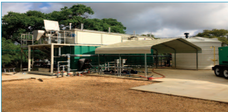
Completed MBR System
