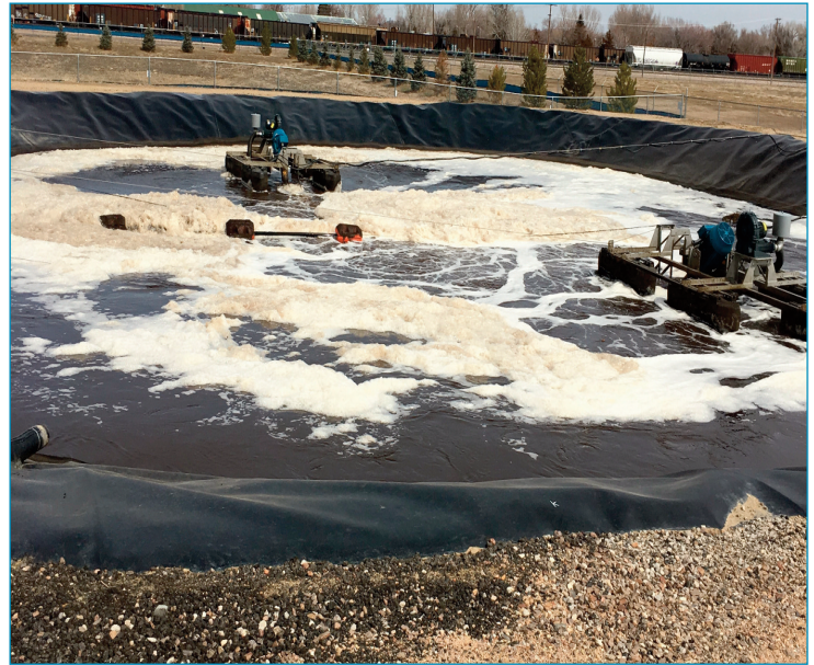
Two New Floating Aerators In Aeration Pond
