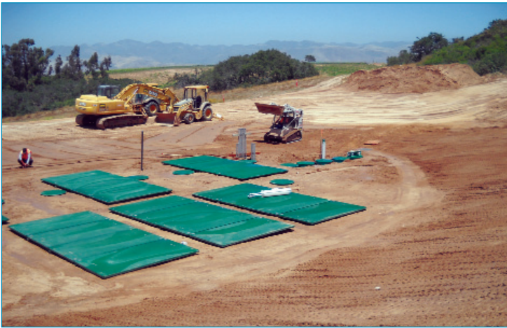
The completed Advantex treatment system installed at or below grade
