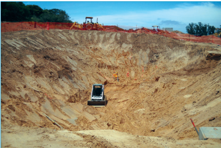
Extensive earth work was required to set the tanks at the correct elevation
