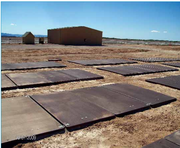
Advantex AX-100 treatment pods installed at grade elevation
