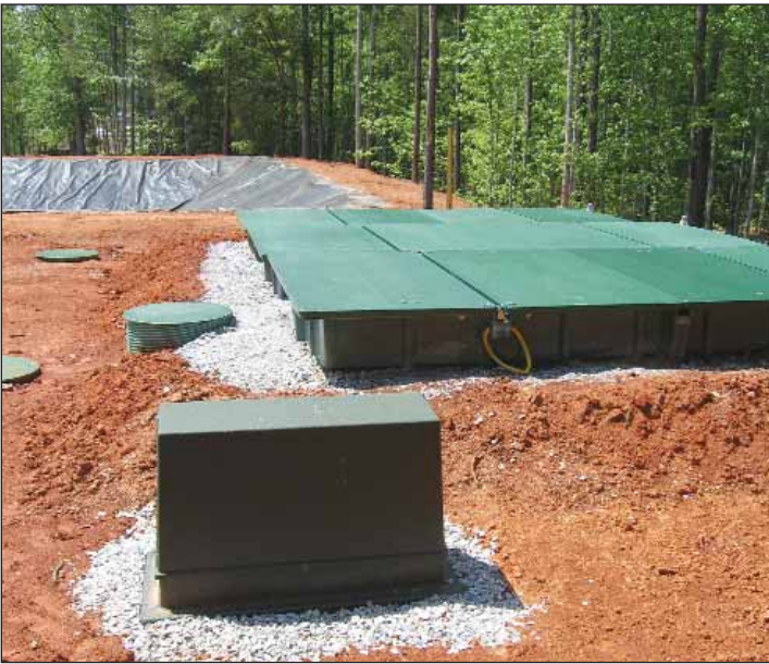
Orenco treatment pods and detention pond
