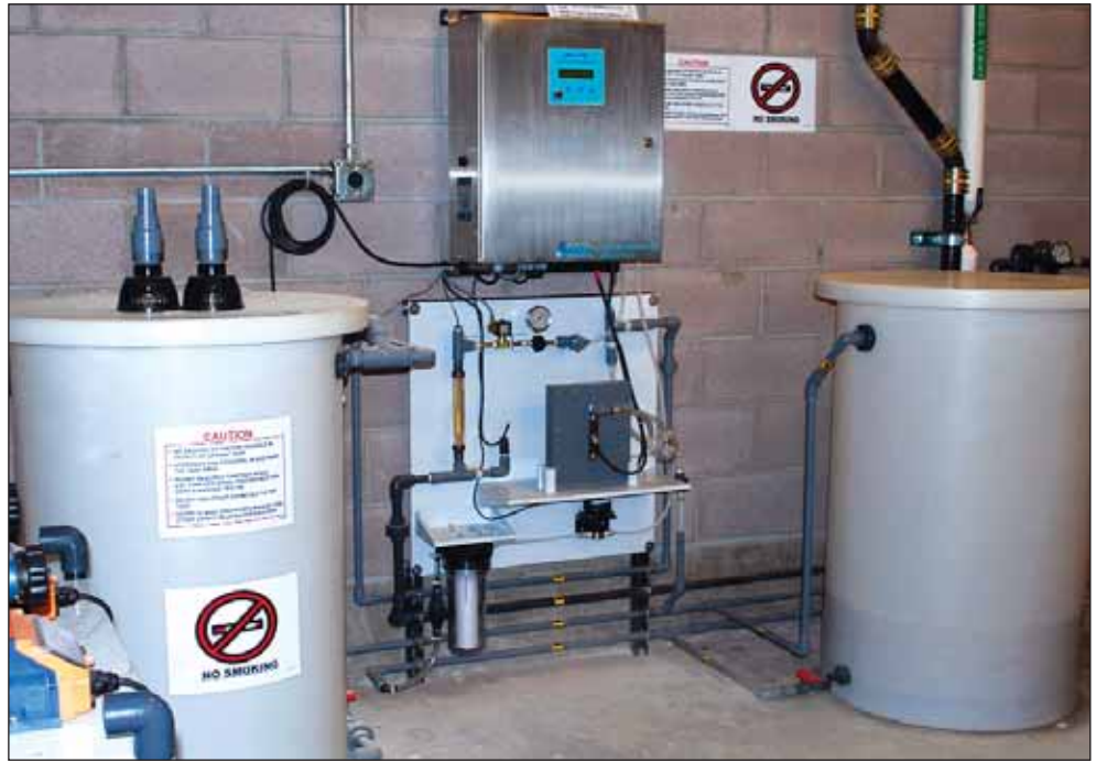
The Miox SAL 40 at UNMH installed in the hospital's utility room
