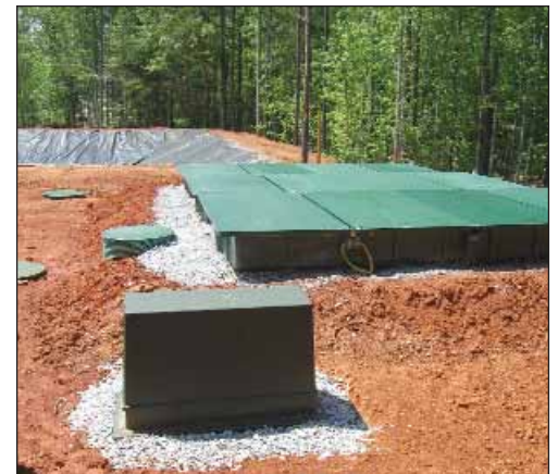
Orenco treatment pods and detention pond
