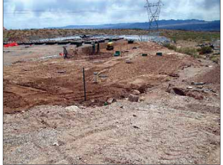
Treatment system area after installation completed
