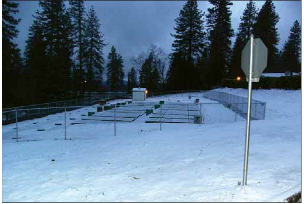
The completed treatment system after a dusting of snow
