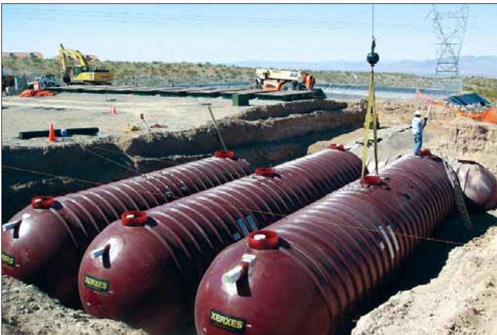
IWS tank installation in foreground
