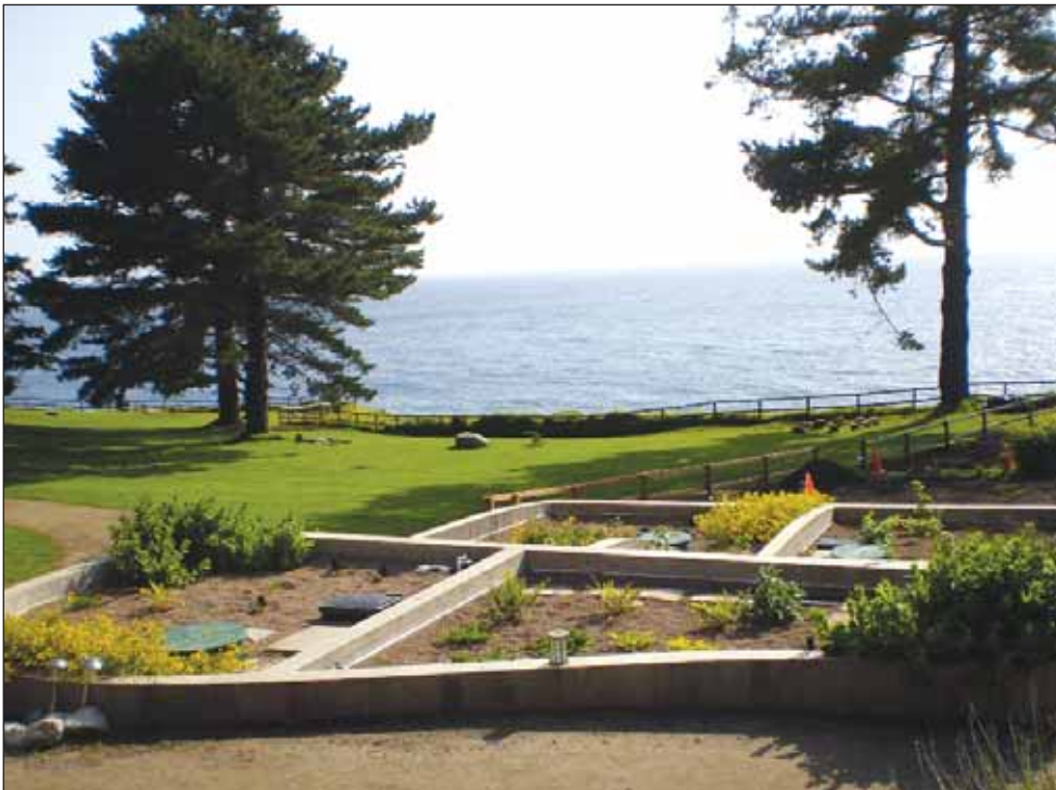
The Living Machine integrated into the Esalen campus
