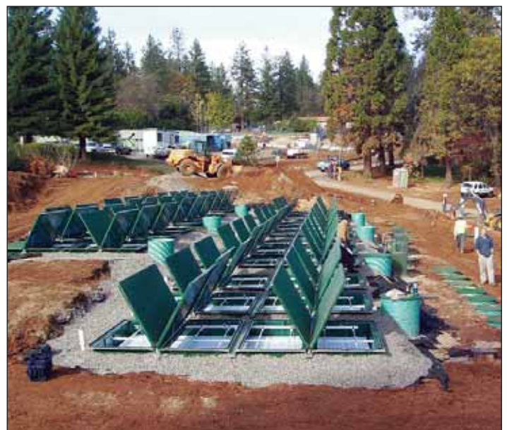
Orenco AX-100 pod open for inspection
