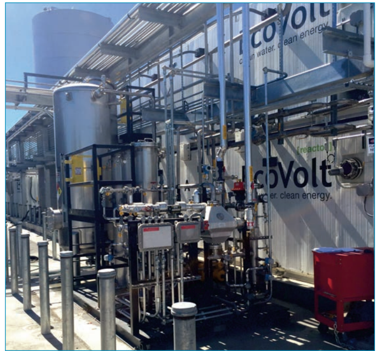
Gas Treatment Skid and EcoVolt Unit
