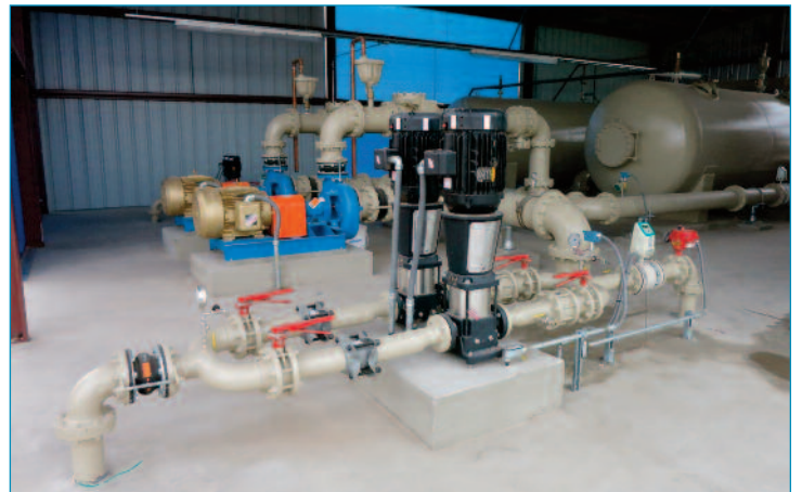
Reclaim Pump System
