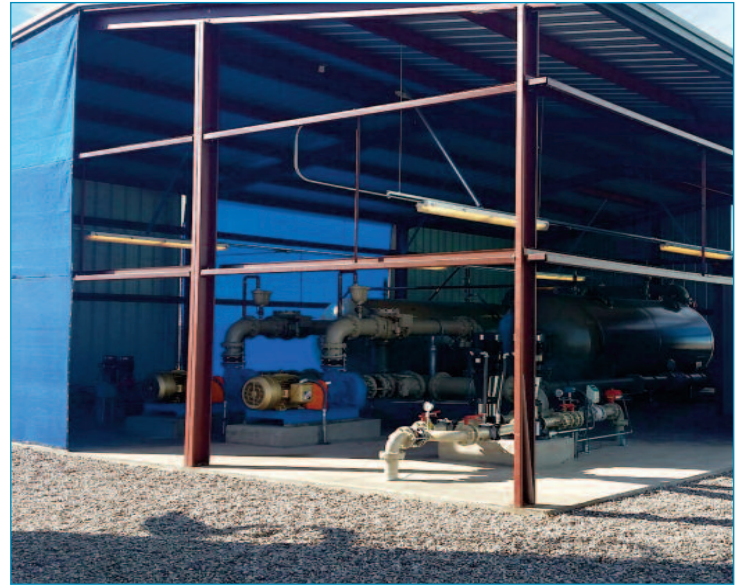
Interior of Treatment Building
