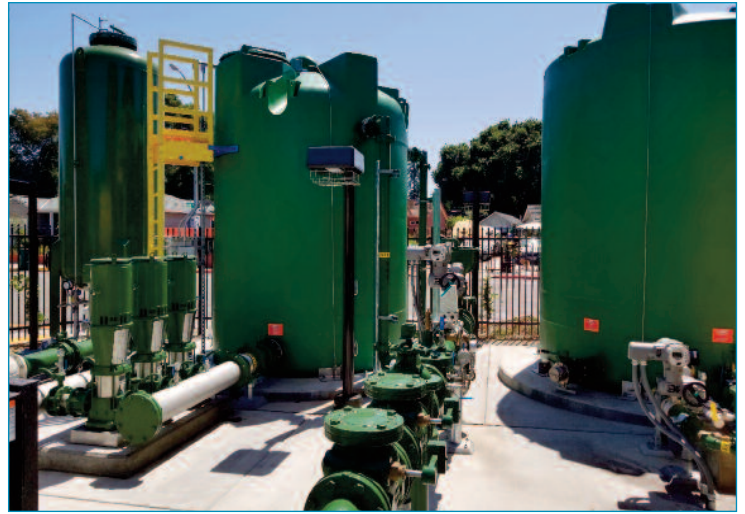
Surge, Blending, and Backwash tanks
