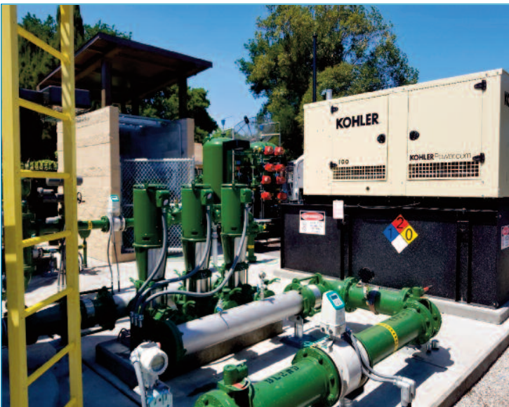
Pumps, piping, and generator
