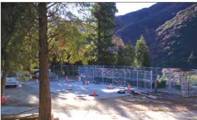
The new wastewater system included primary and secondary treatment
