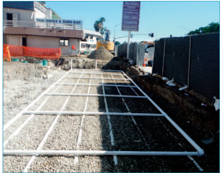
North parking lot drainfield pipe
