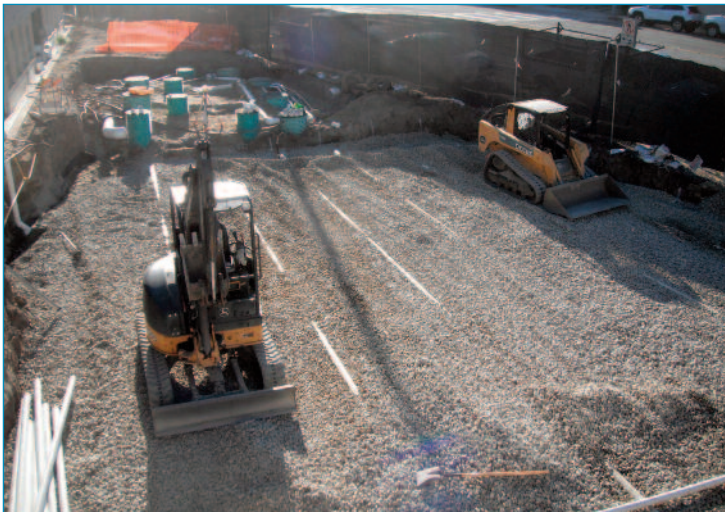
South parking lot leachfield and tank risers
