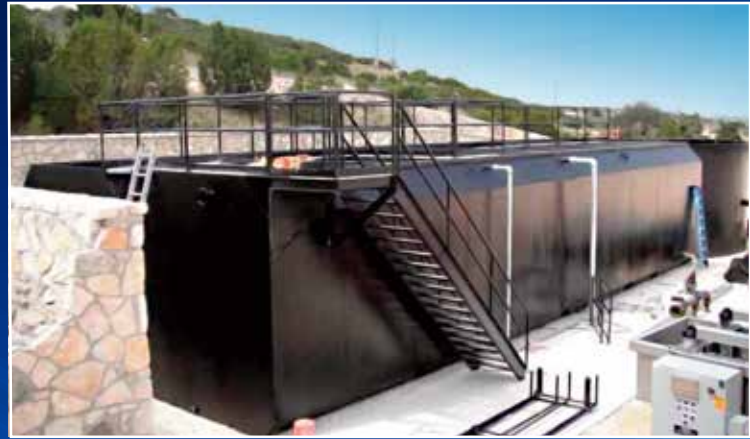
This Wastewater treatment plant in Kendall County, Texas is hidden from view by a retaining wall and below grade foundation.
