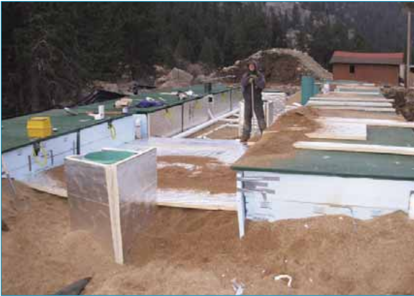
The treatment pods required insulation to protect from freezing temperatures
