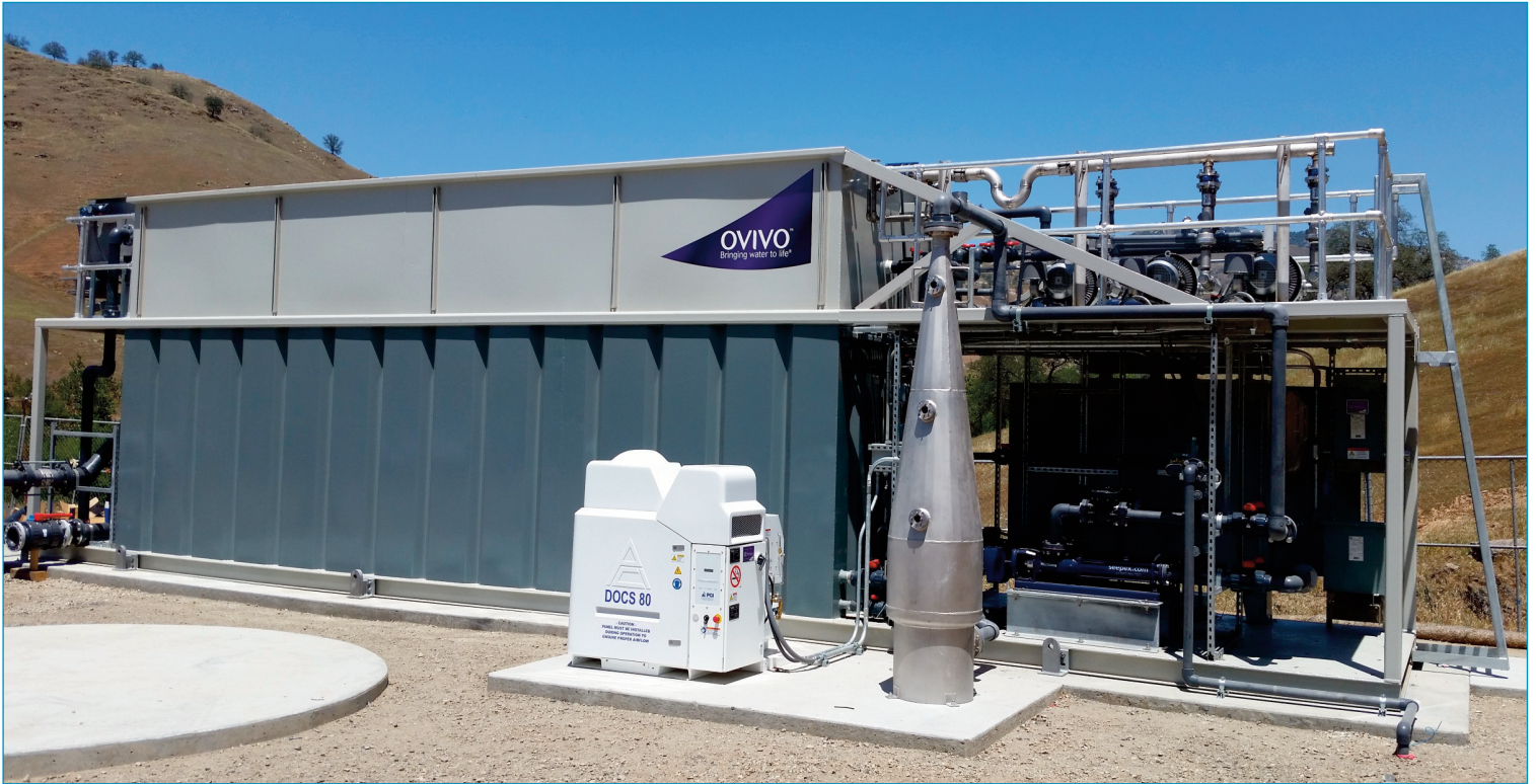
microBLOX unit installed
