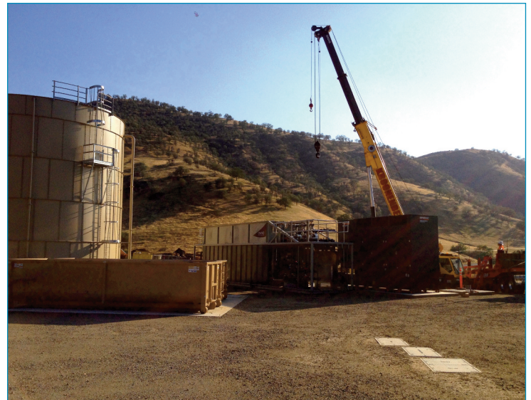
Water Tank, microBlox, and Generator
