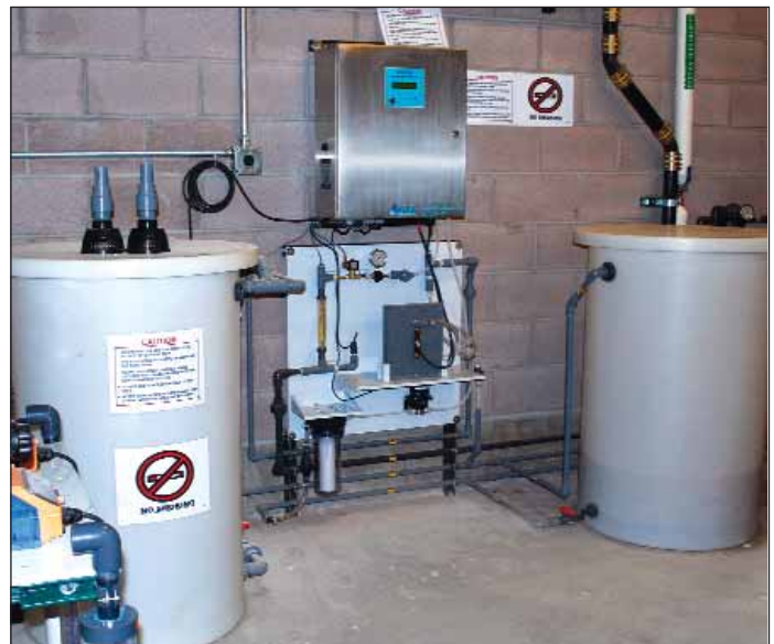
The Miox SAL 40 at UNMH installed in the hospital's utility room
