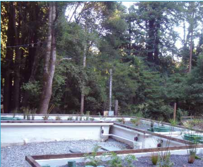
Living Machine® System treatment cells
