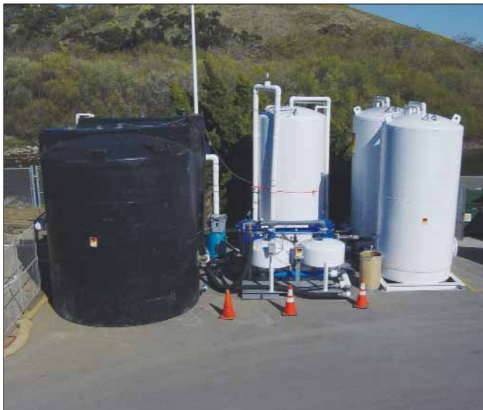
Pure Effect Dewatering Treatment Train
