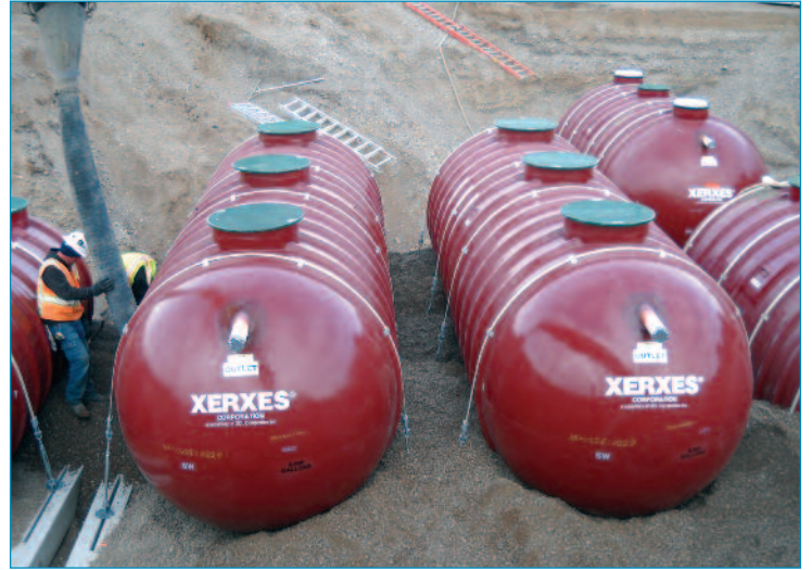
The two center tanks are the IWS Upflow Filters
