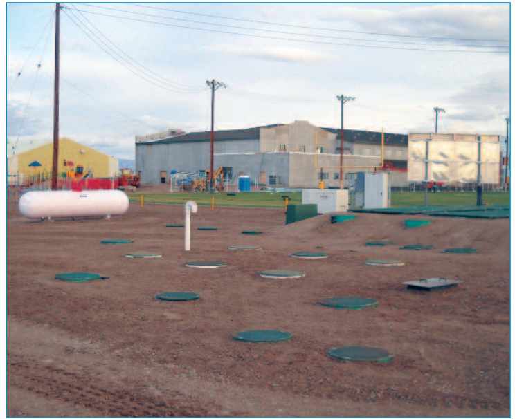
View of the completed treatment system
