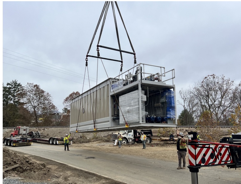
An IWS BluBox unit being deployed.
