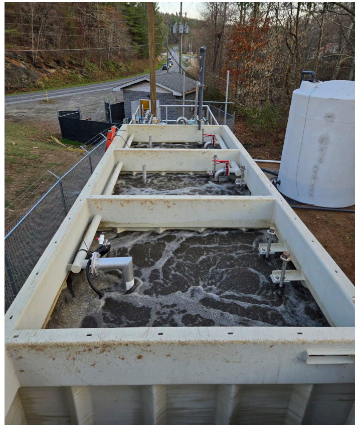
An IWS BluBox unit treating wastewater in the town of Spruce Pine, North Carolina, after Hurricane Helene.
