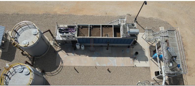
An IWS BluBox unit deployed on site.
