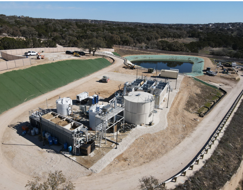
An IWS installation in the Hill Country of Texas.
